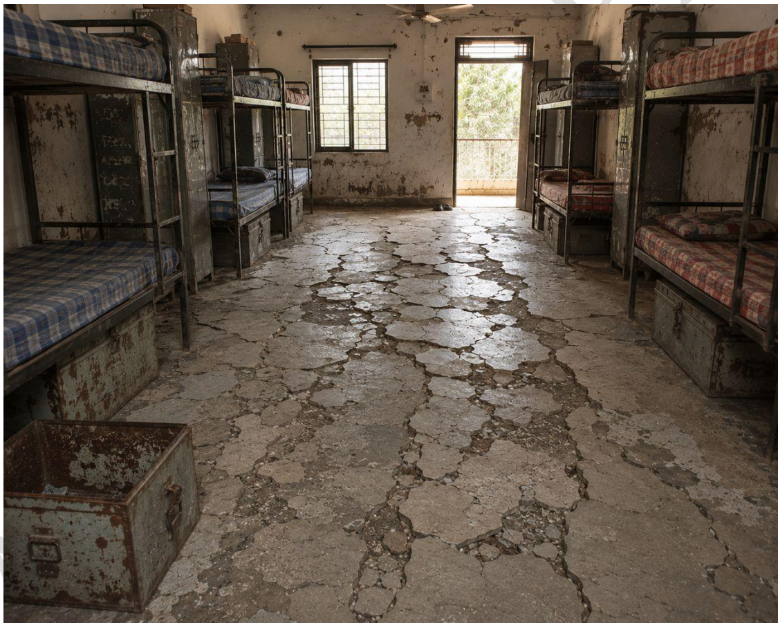
Fig. 1 – Photo showing the damaged floor and boxes in the dormitory.
